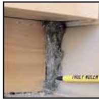
In cabinetry cracks, both inside and outside of units.
