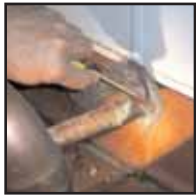
Around incoming gas and water lines.
