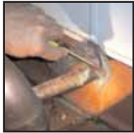
Around incoming gas and water lines.
